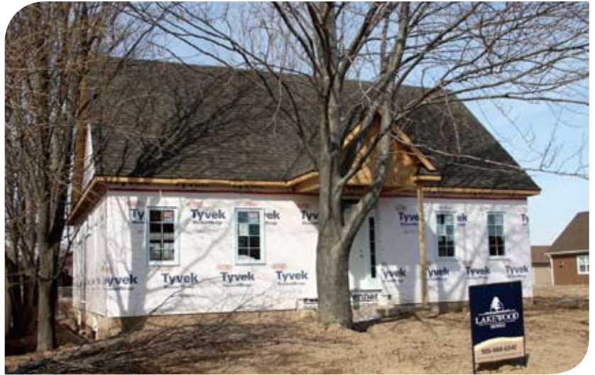
This expandable bungalow is under construction right now and can be ready for you in May
